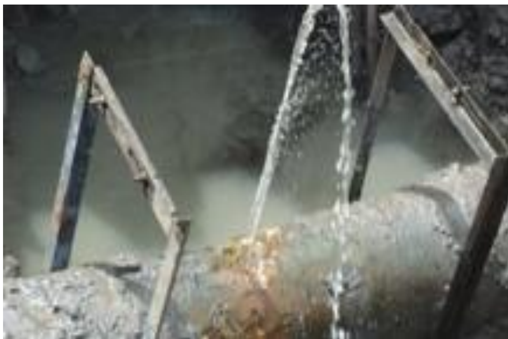
Figure 1: Water fountain from the 24" Bomu-Bonny corroded pipeline facility at 12 O' clock position in Andoni, Rivers State
